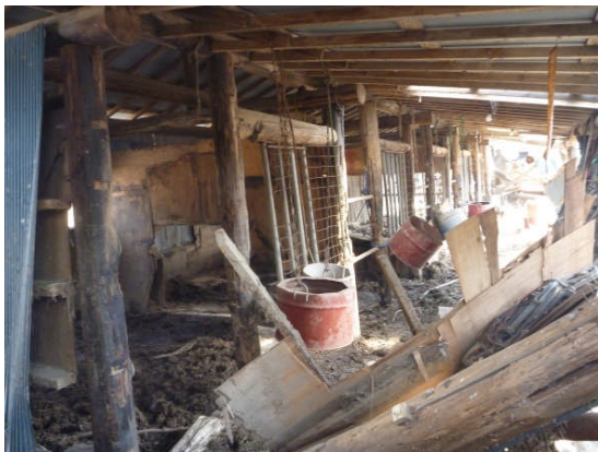
(Photograph 2) Damage to horse stables by the earthquake
