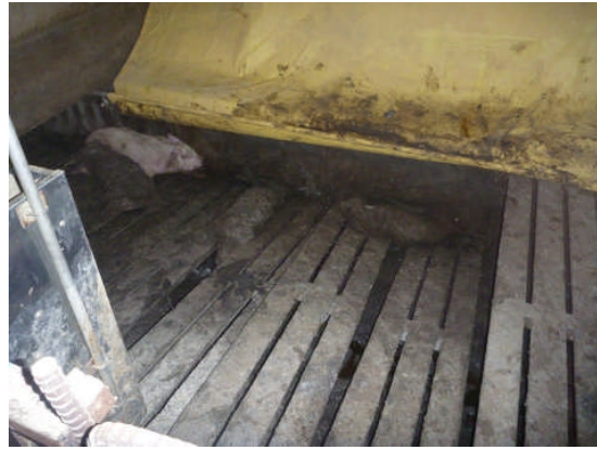
(Photograph 43) A part of the floor was damaged by the earthquake. Although it was not possible to count the accurate number of dead pigs, over 400 bodies were found.
