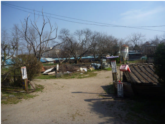
(Photograph 29) The buildings on the right and center of this photo had collapsed. Nobody has entered the hen house at the rear because it was dangerous.
