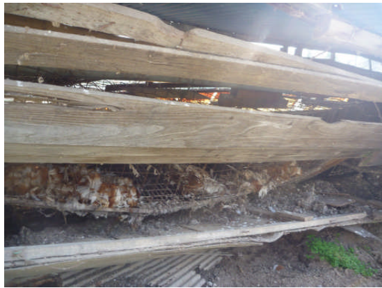
(Photograph 28) This hen facility had totally collapsed; therefore, only a brief inspection was possible. The cackling of hens could not be heard in collapsed facilities like this one.
