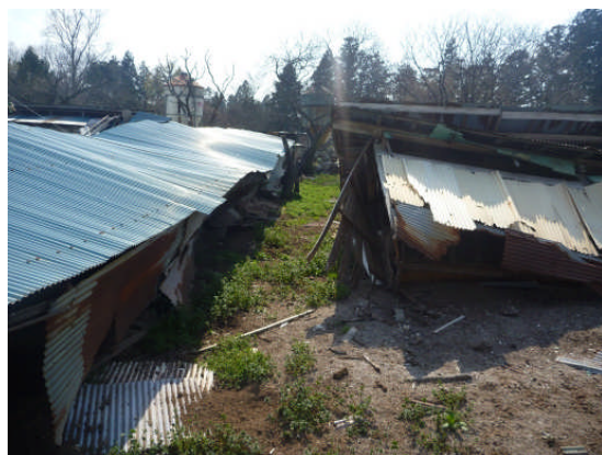
(Photograph 30) This hen house was about to collapse. Crows could no longer be heard in this area.
